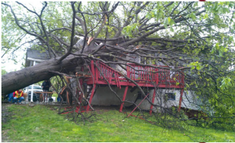
Damage from Tornado, 2011.
